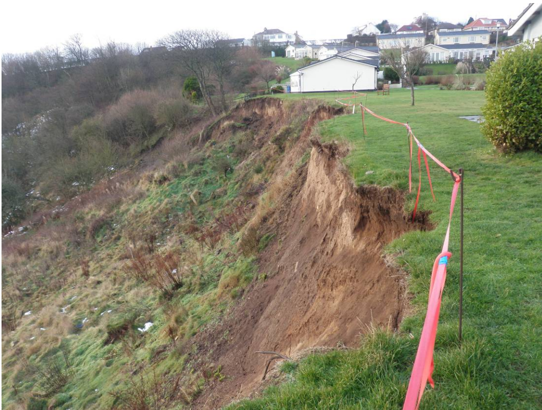
Plate 8 Cliff recession at Knipe Point Headscarp (13 th December 2010)
